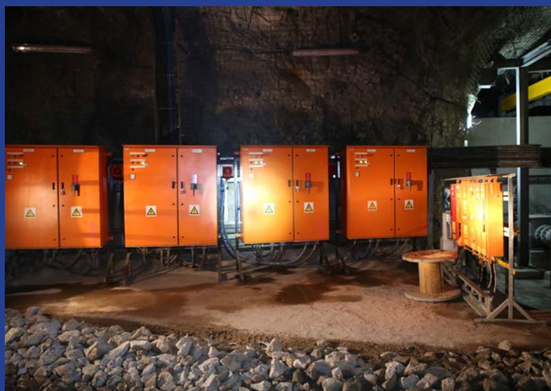
Ramp 2 – 175ml Newly commissioned Pump Chamber.
